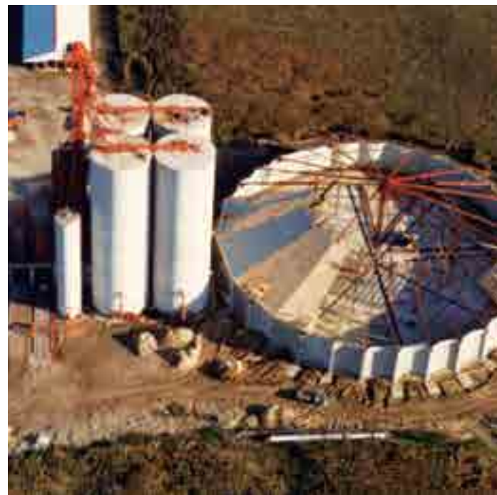
Top: The centre support tower of the Melbourne grain storage building is being loaded on the truck at the Steelway plant. Bottom: Aerial view of the Melbourne project under construction, 1982.
