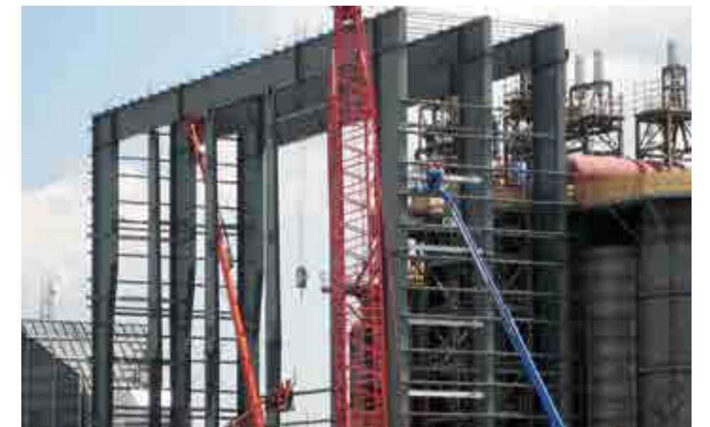
The Halton Hills Generating Station in Halton Hills, Ontario.
